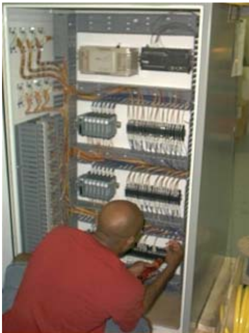
Inside of cabinet during checkout. View of PLC, temperature controllers, and output solid state relays.
